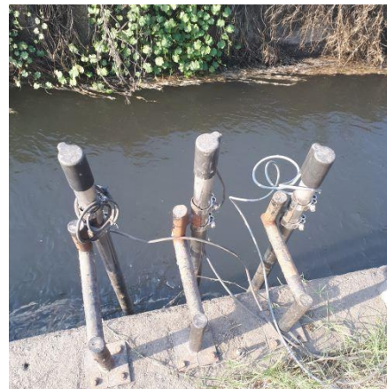
FG116: Sensores de control
